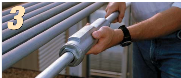
Thread the next length of conduit into the other end of the fitting and tighten. You're done!
